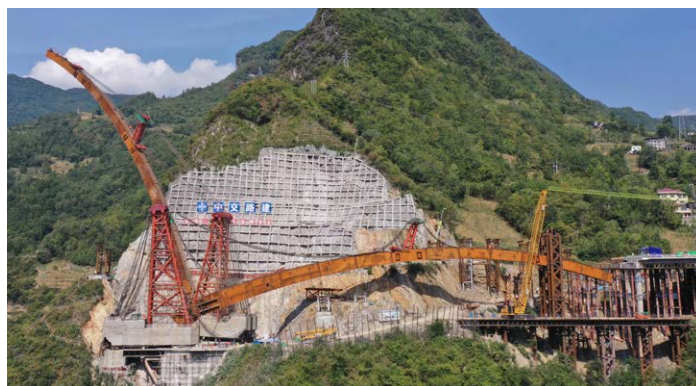
The Liaozi Grand Bridge provides the final link along the Chengkou Expressway, connecting every county in Chongqing to modern convenient transportation.
